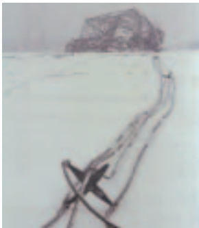
A downed hydro tower and power line, damaged by the 1998 ice storm in Quebec and Ontario.
